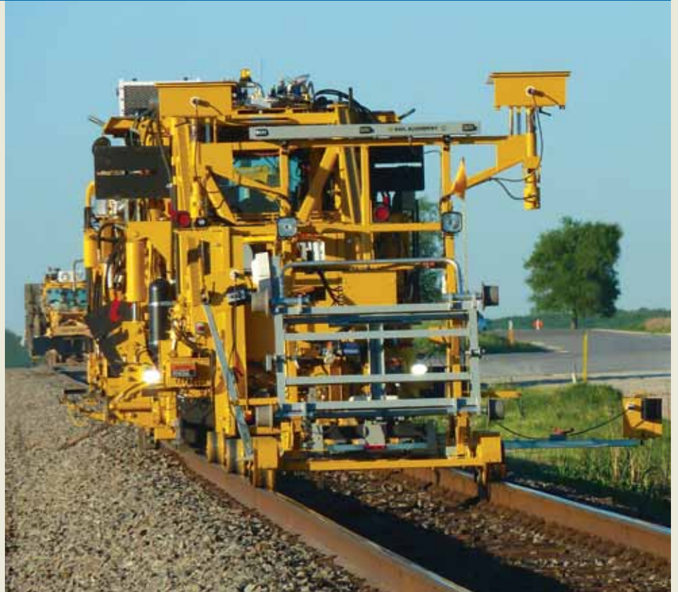
The first drone tamper on BNSF includes a main tamper with a robot-like framework at the front while a trailer comes up from behind. The main tamper controls the trailer with remote control technology.
